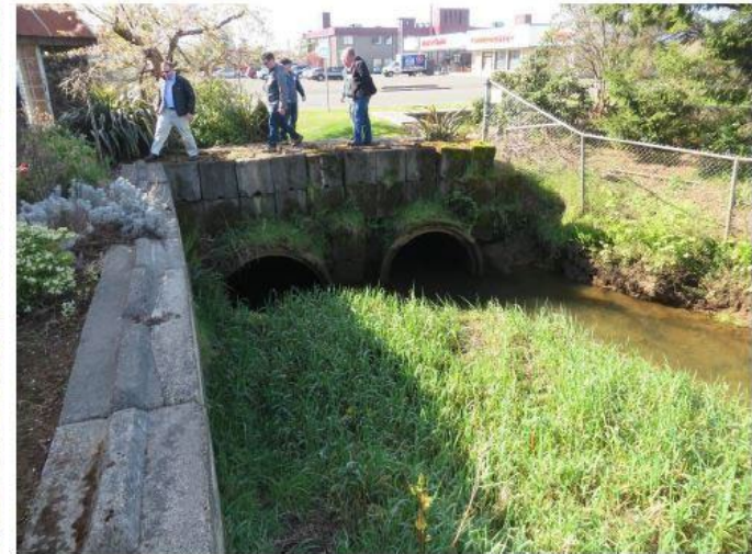
FRY CREEK - CULVERT CONSTRICTIONS
